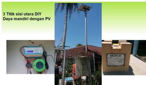
Figure 7 Remote station of Groundwater Level Sensor
