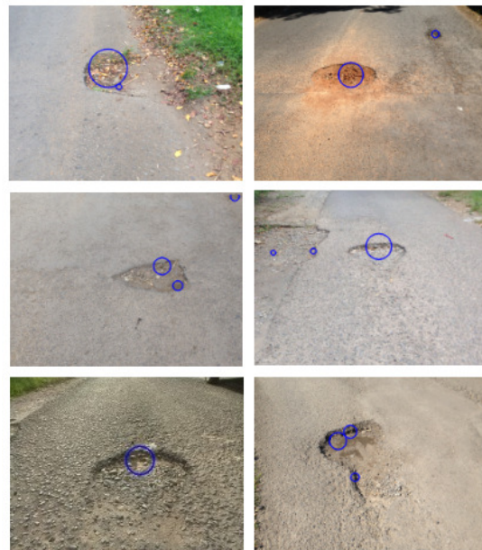
Figure 7: Examples of detected potholes in asphalt pavement images.
