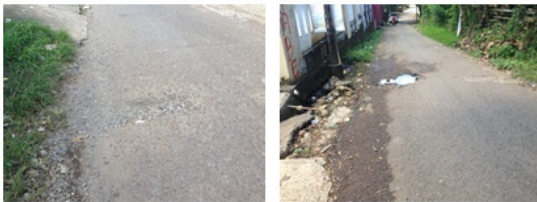
Figure 8: Example of non-detected pothole.
