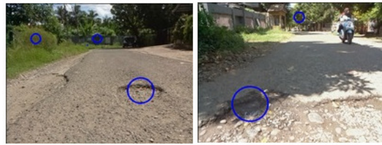
Figure 10: Pothole detection results by increasing \alpha \approx 90^\circ . By increasing the \alpha angle, means it the camera would be pointed more upward, but objects outside the road that has same visual characteristic with the potholes could be detected as a pothole either.
